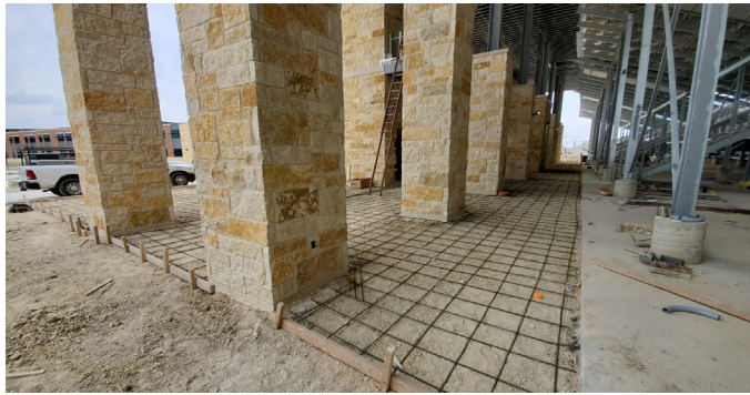
Site: Flatwork being prepped for place and finish at football bleacher area.
