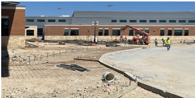
Site: Concrete sidewalks being prep for place and finish near the Auditorium entrance.
