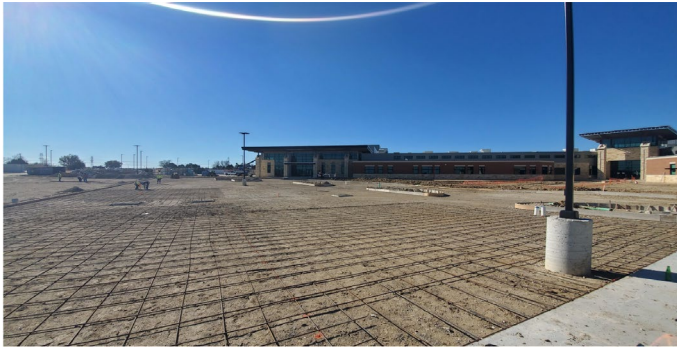
Site: South area concrete parking lot and sidewalks being prepped for placement.
