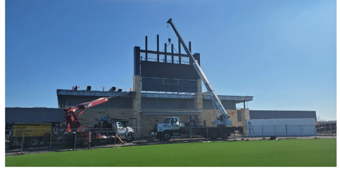
Site: Football Stadium scoreboard and video display board being lifted into place.
