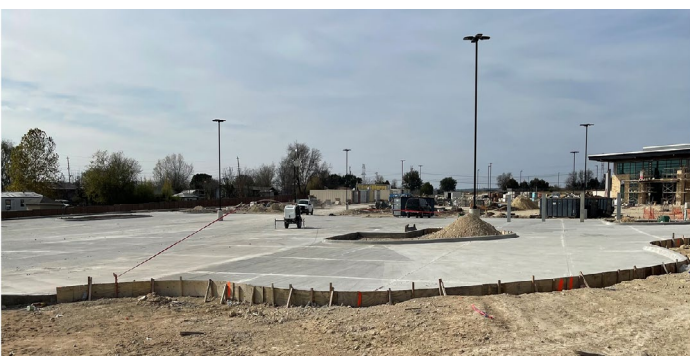
Site: Concrete paving placed and finished at south side of Area MNP.
