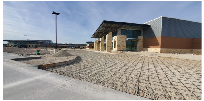
Site: Concrete paving prep for place and finish on the south side of Area MNP.
