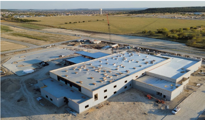
Exterior: Drone view; Lightweight concrete roof at low area 3 and area 6, decking on area 5.
