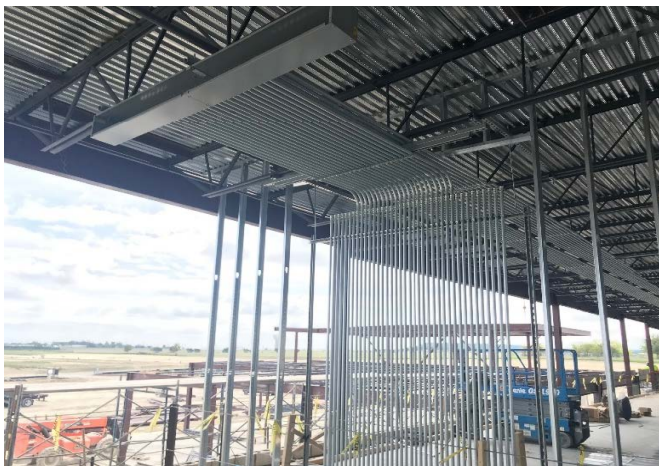
Interior: Area 2 and 3 conduit runs for electrical.
