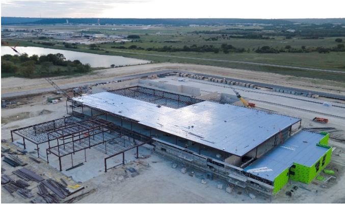
Exterior: Drone view; steel structure install in Area 1; roof decking area Areaa 5 & 6
