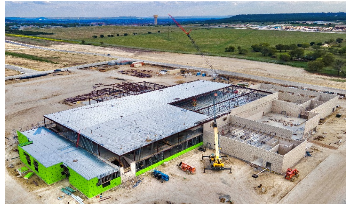
Exterior: Drone view; topped out CMU Area 4; framing and outer sheathing Area 3
