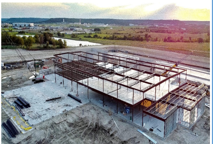
Exterior: Drone view form Northeast; Area 3 & 6 steel installed, slab on metal deck installed.
