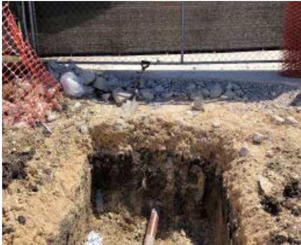
Field House Water: Old water line from field house is capped at back at Nolan MS.
