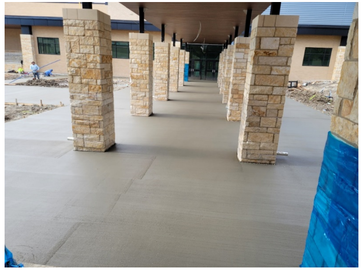
Area D&T Courtyard: Aluminum canopy installation complete. Concrete flatwork installation in progress.
