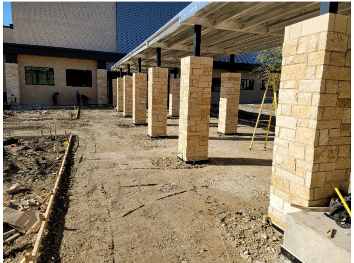
Area D&T Courtyard: Aluminum canopy installation and concrete flatwork prep in progress.
