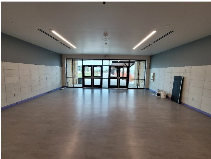
Area C: Cleaning and base installation in progress. Turnover to KISD on 11/14/22.
