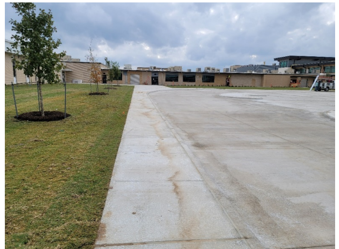
Area M&N Courtyard: Landscaping, aluminum canopy soffit, and exterior lighting installation in progress.
